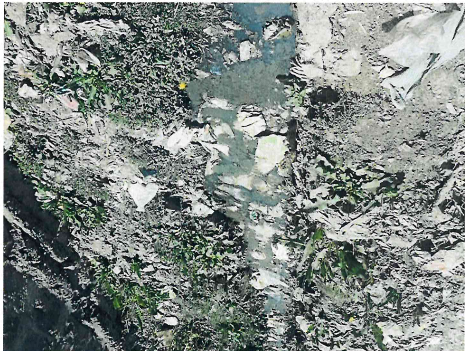
Figure 6-12: Poor drainage channel in Captain Centre
