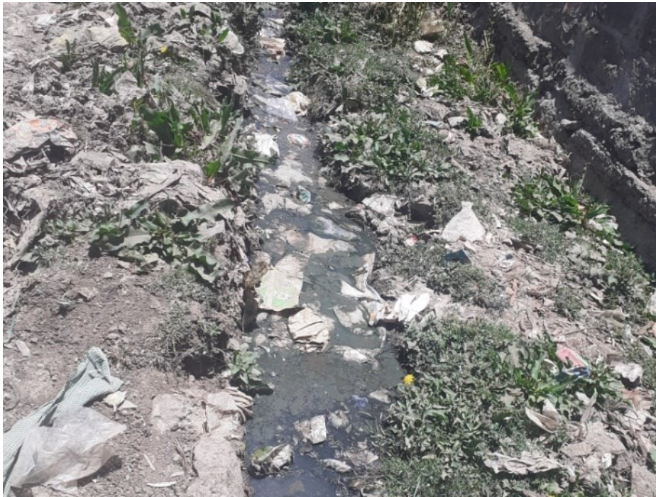
Figure 6-12: Poor drainage channel in Kaptain Centre
